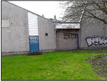
Photograph 13: Building with PRFs via gaps behind wooden soffit box adjacent to the site
