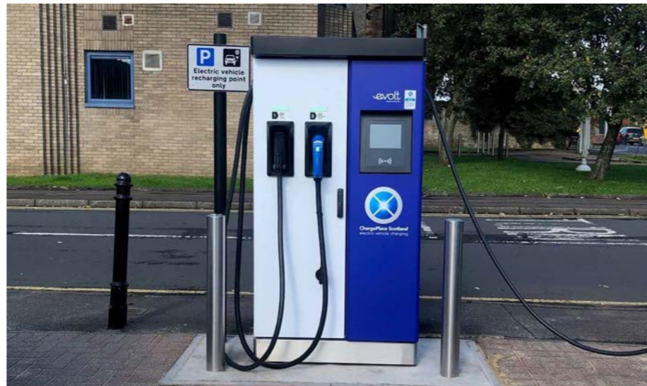
Electric vehicle charging points
